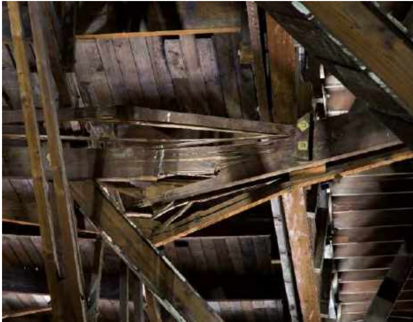
Figure 5. Broken top chord near roof monitor at top of truss
