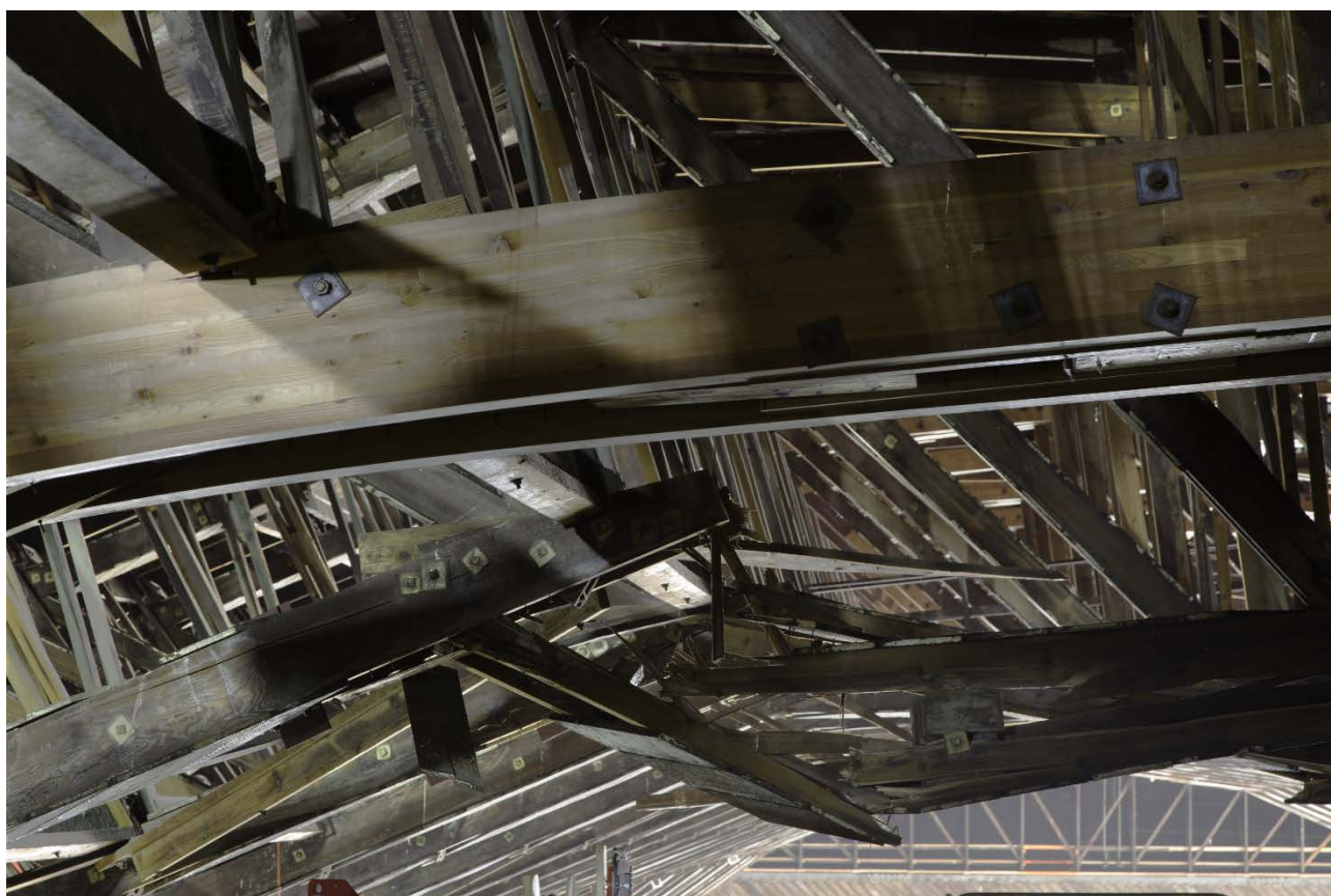
Figure 6. Broken bottom chord near top of truss.
