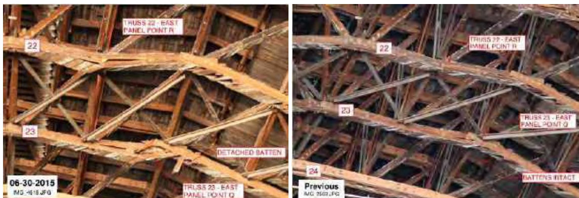
Figure 2. Truss damage progress at Trusses 22 and 23 East near Panel Points R and Q.
