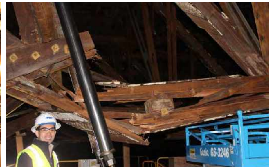
Damaged chord member viewed from access tower
