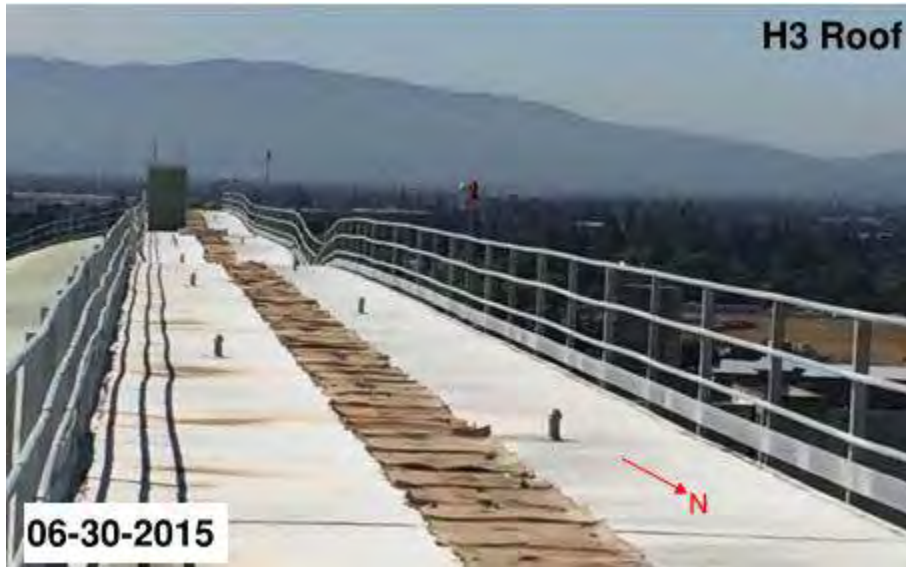
Figure 3. Damage observable at ridge line from building exterior.
