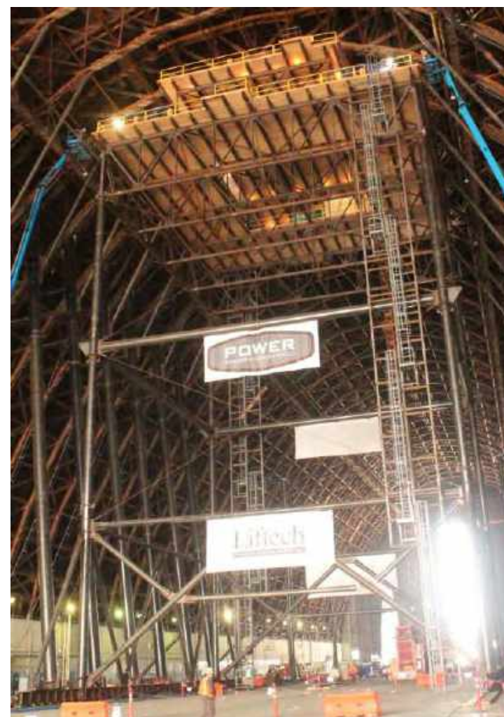
Movable access tower
