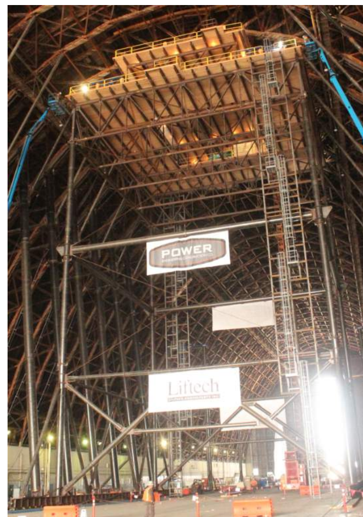
Movable access tower
