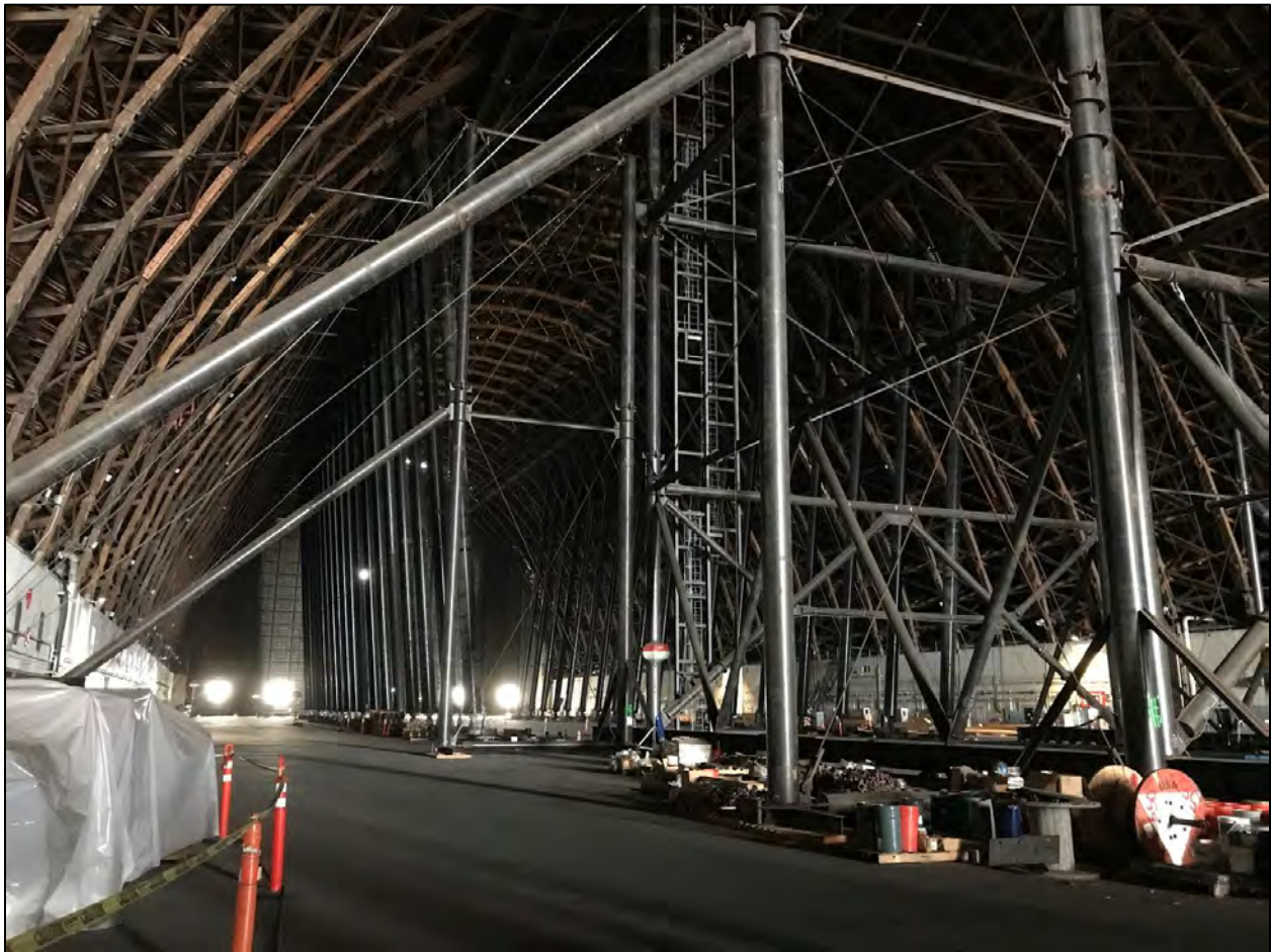
Photograph 2: Interior volume Hangar 3 showing the hydraulic jack system which runs the length of the main structure and the repair scaffolding deck at center.
